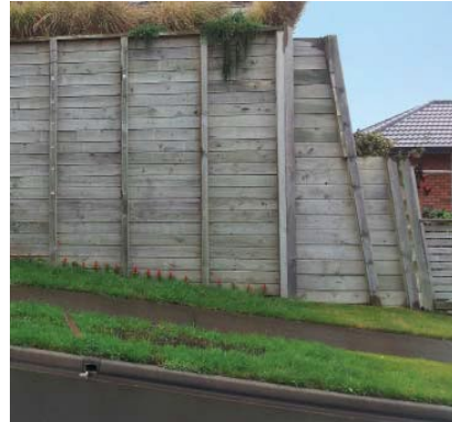
Example of an out-of-scale retaining wall devoid of planting which detracts from the amenity of the streetscape.
