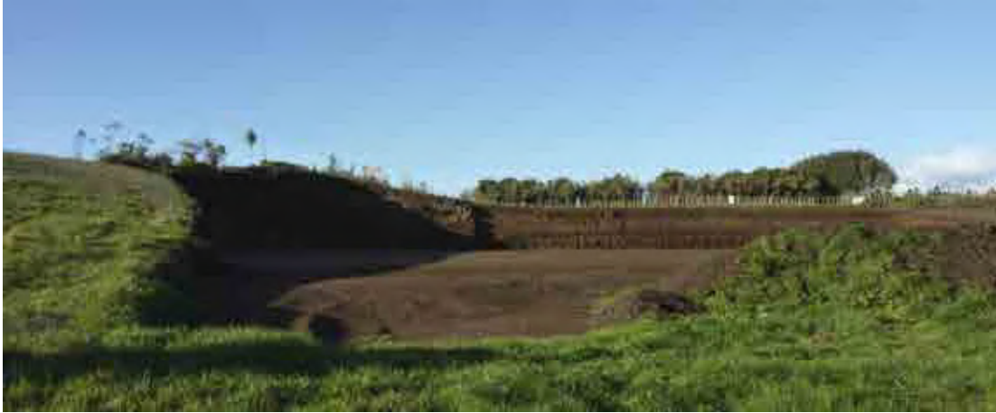
Figure 11: Exposed bank cutting on the boundary of southern boundary of Property 1, facing south towards Property 6.
