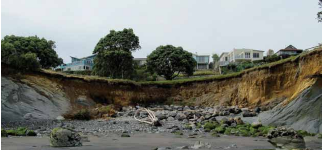
Coastal Erosion at Motukari Reserve, Onaero
