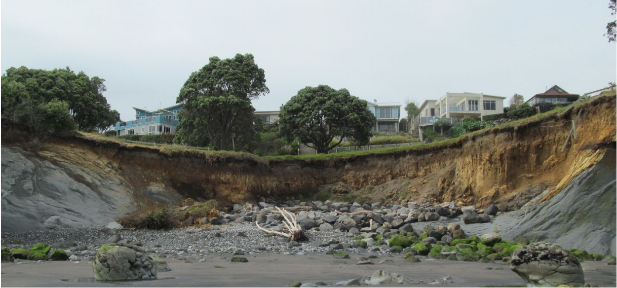
Coastal Erosion at Motukari Reserve, Onaero
