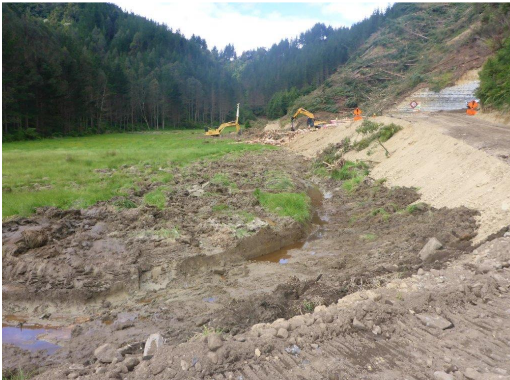
Figure C 25: Site Ea30, Mimi River catchment. Fill is proposed in this valley. The cut-off drain on true right of the valley has been by recent logging. The main stream is on true right of the valley is not affected by the Project.
