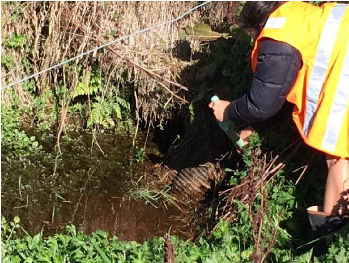
Figure 4: Drainage coil discharging to waterway
