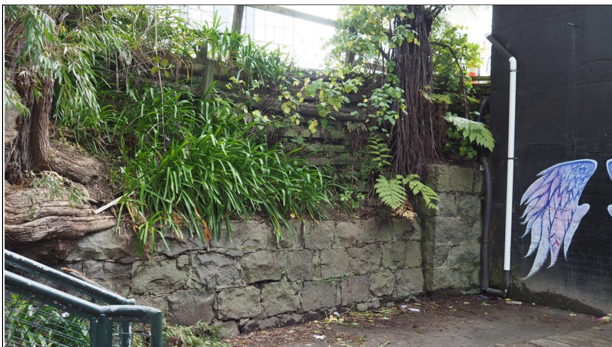
Figure 14: Remnant section of stone railway embankment, retained eastern boundary of project area above (Image: Ivan Bruce, 2019).
